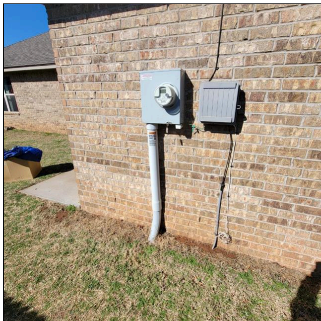
9.0 Item 1 (Picture) Electrical Meter
